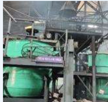
Organic Mixing (Slurry Tank)
